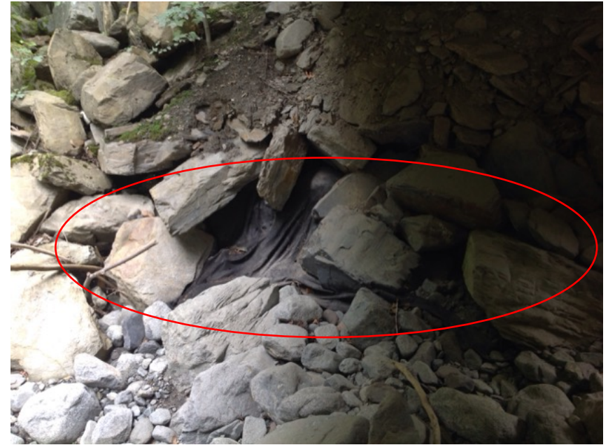
riprap scour downstream right bank
